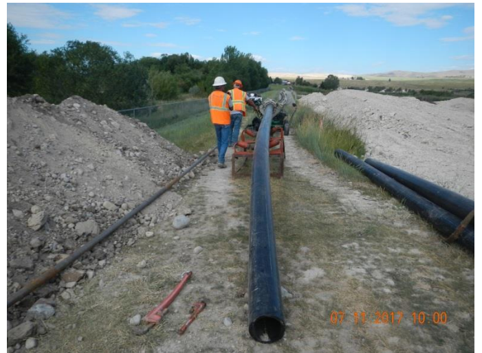
Figure 4 – Fusion Welding HDPE for Pulling Under Kerr Dam Road; Potable Water Main
