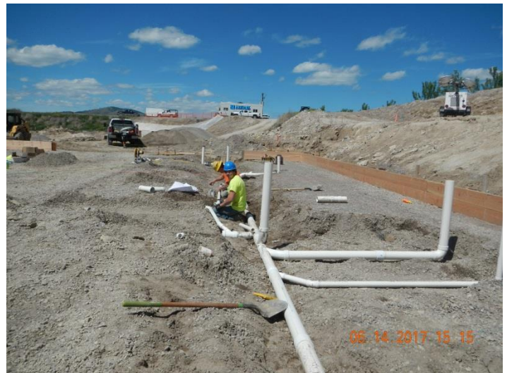
Figure 4 – Below Slab Piping – Control Bldg. Basement
