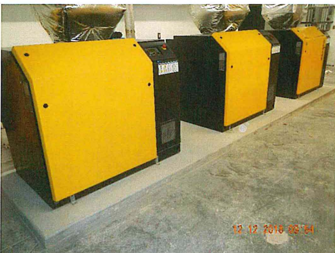
Figure 11 - Digester Blowers; Ready for Operation
