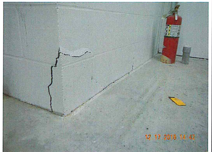
Figure 6 - Interior Masonry Crack Needing Repair
