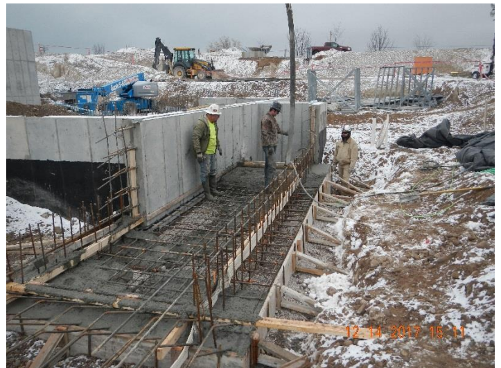
Figure 4 - UV System - Flow Channel Floor
