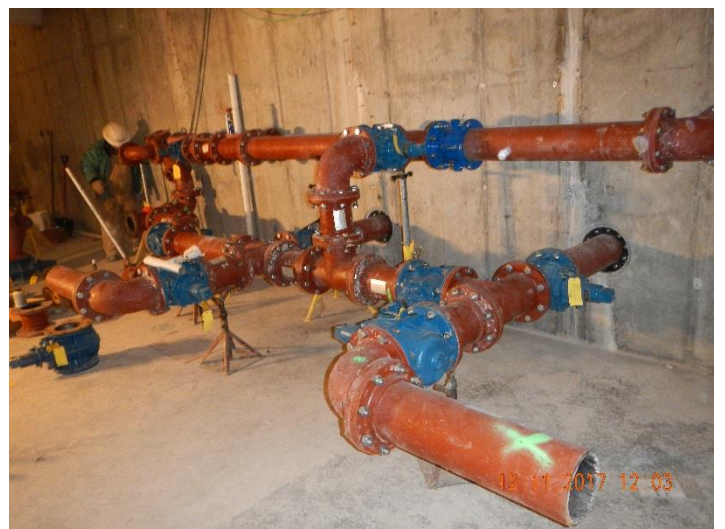
Figure 6 - Control Building Process Pipe
