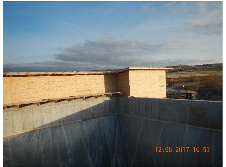
Figure 8 - Inside Digesters - Seep Repair, Heating Provisions
