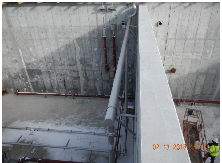
Figure 8- Digester 1; Aeration Piping
