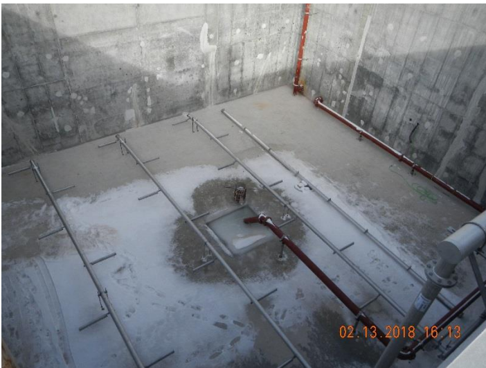
Figure 7 - Digester 1; Aeration Piping & Sludge Piping
