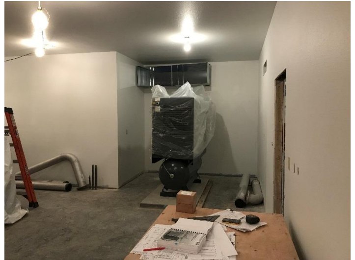
Figure 5 - Cntrl Bldg.; Compressor For Digester Mixing System
