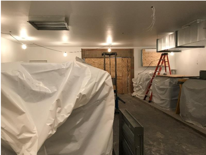
Figure 6 - Control Bldg. Blower Room
