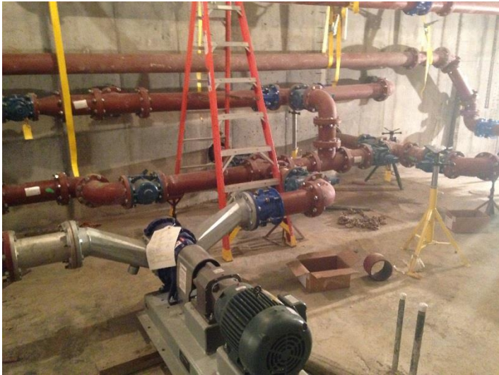
Figure 5 - Digester Process Piping
