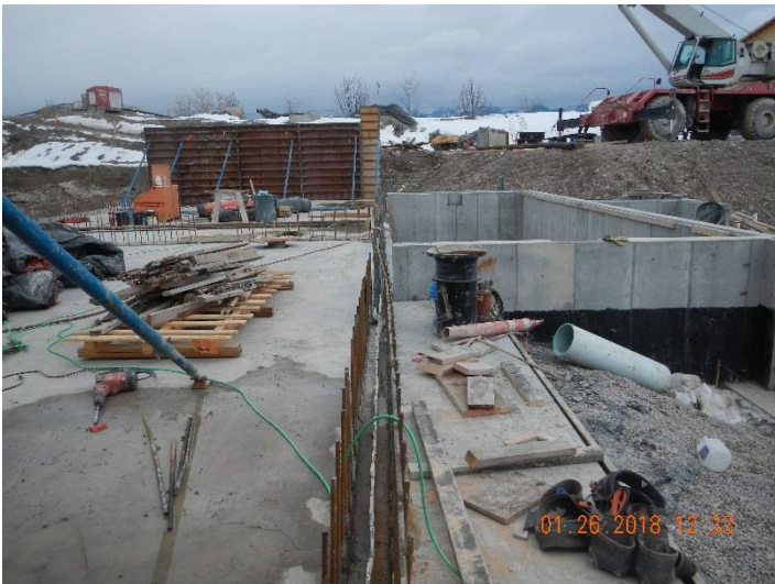
Figure 3 - Post EQ Floor & Pipe Gallery
