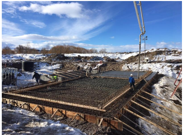
Figure 2 - Post EQ Tank Floor
