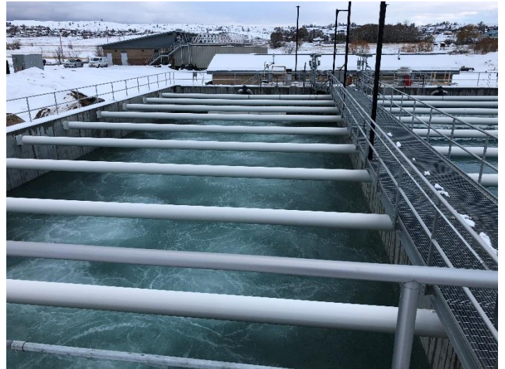
Figure 2 – SBR Tank #1 With Aeration and Mixing in Operation
