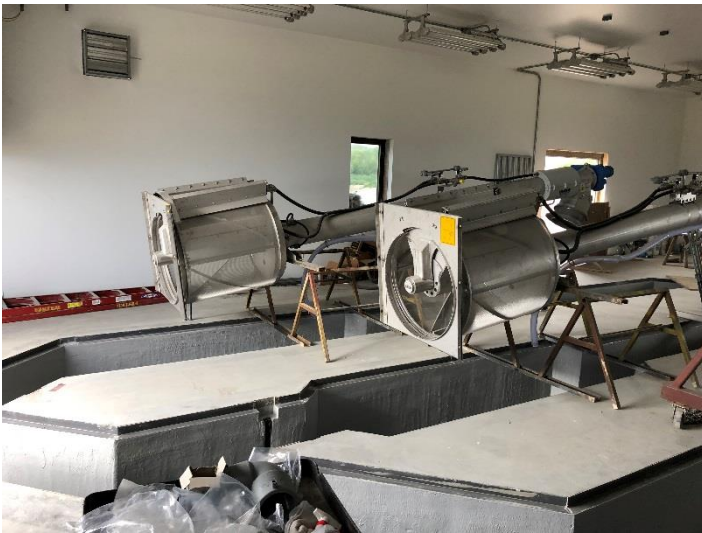
Figure 3 - Headworks, Influent Screens
