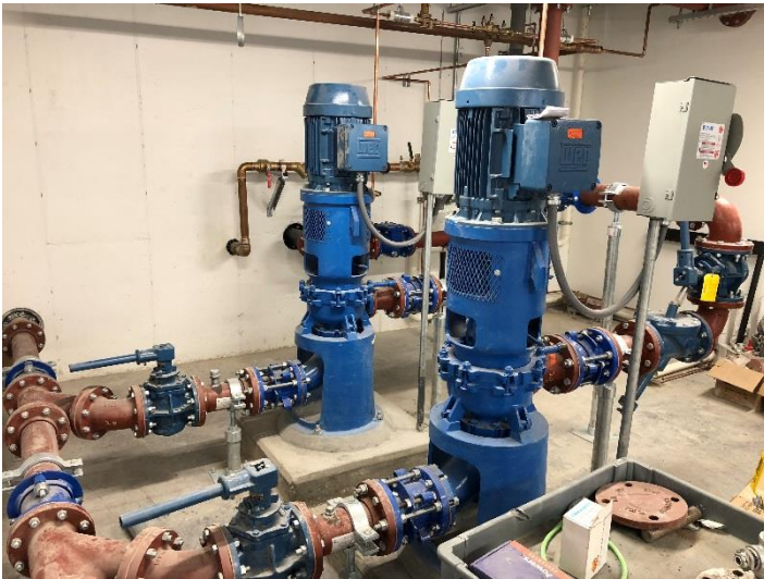
Figure 1 - Headworks Building, Grit Pumps
