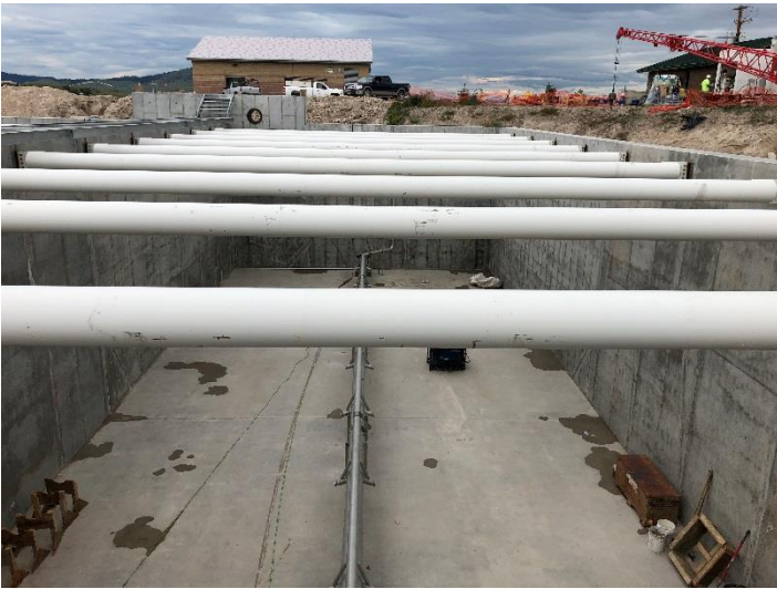
Figure 7 - SBR Equipment; Aeration Header
