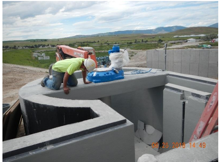
Figure 2 - Grit Chamber, Paddle Drive Installation
