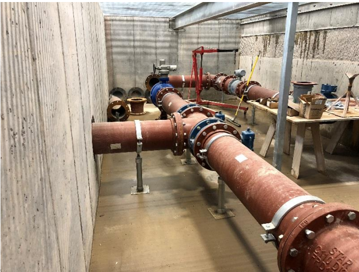
Figure 9 - UV Bldg.; Outlet Control Piping
