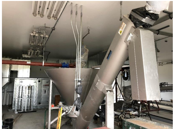
Figure 4 - Headworks - Grit Washer
