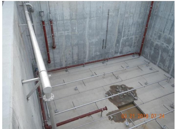
Figure 9 - Digester Aeration and Mixing Piping
