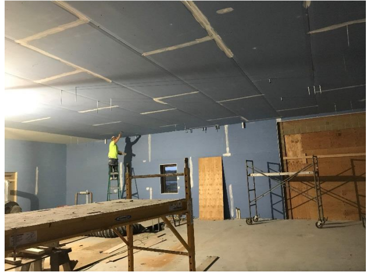
Figure 2 - Interior/Main Floor Headworks Bldg.
