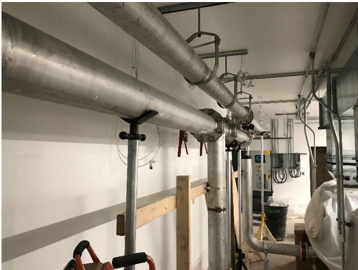
Figure 8 - SBR Blowers - Aeration Piping
