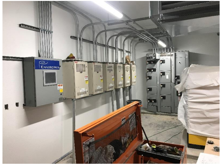
Figure 7 - Electrical; Process Blower Equipment
