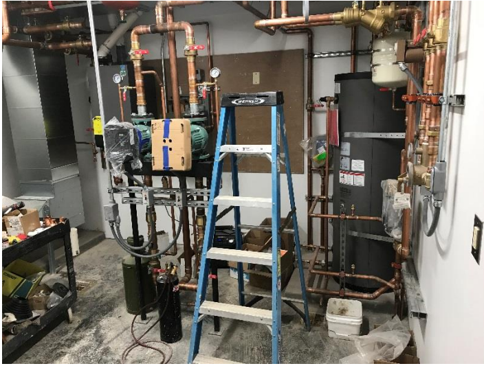
Figure 6 - Control Bldg; Heating/Boiler System
