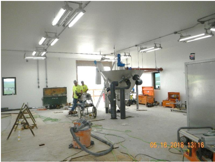
Figure 1- Headworks Equipment, Grit Washer
