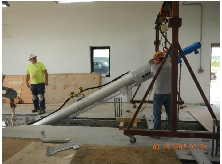
Figure 2 - Headworks Equipment - Influent Screen
