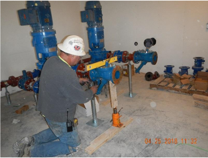
Figure 1 - Grit Pumps, Headworks Basement
