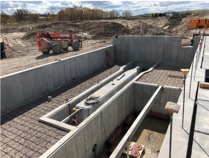
Figure 3 - UV Channels; Outlet Control Vault
