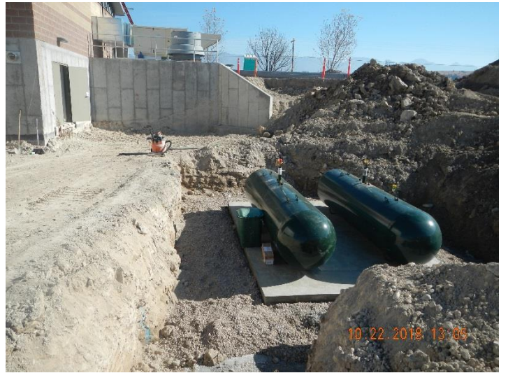
Figure 4 - Control Building, Propane Tanks
