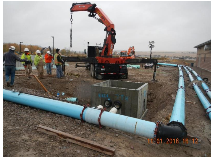
Figure 9 - Force Main Collection Vault (Bypass Piping)
