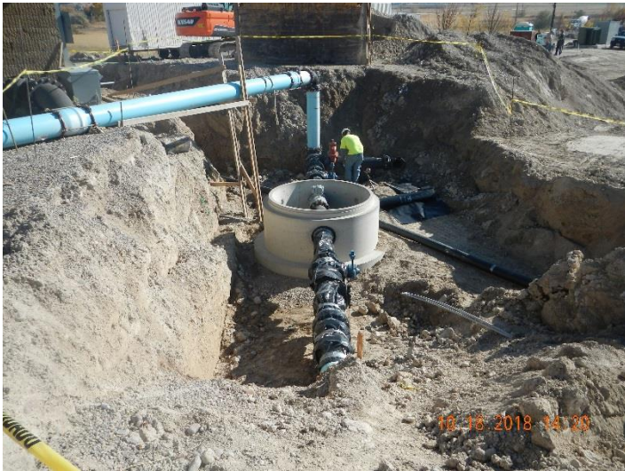
Figure 8 - Ducharme Force Main, Meter Vault & Bypass
