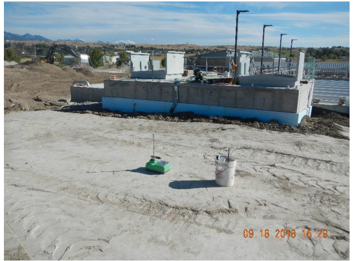
Figure 2 - SBR Inlet Vault; Flow Control Valve Housing
