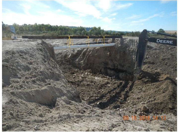
Figure 8 - Temporary Pipe Support; 24" Eff. Pipe Below
