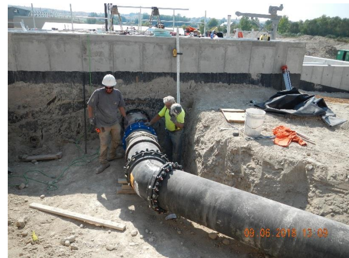
Figure 4 - Influent Pipe Connection to SBR Inlet Vault
