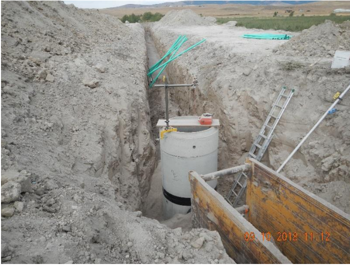
Figure 7 - 24" Effluent Pipe to River
