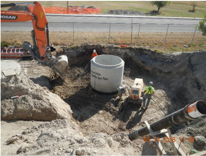
Figure 1 - Riverside Lift Station; Flow Meter Manhole (1 of 3 vaults)
