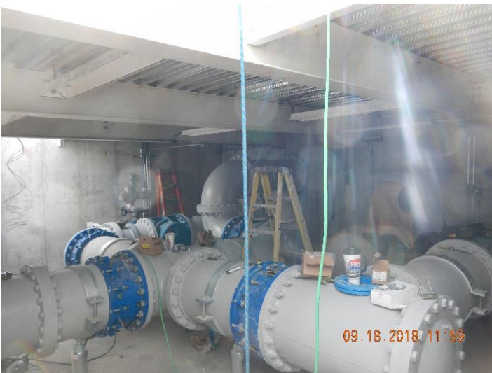
Figure 3 - Process Piping Inside SBR Inlet Vault
