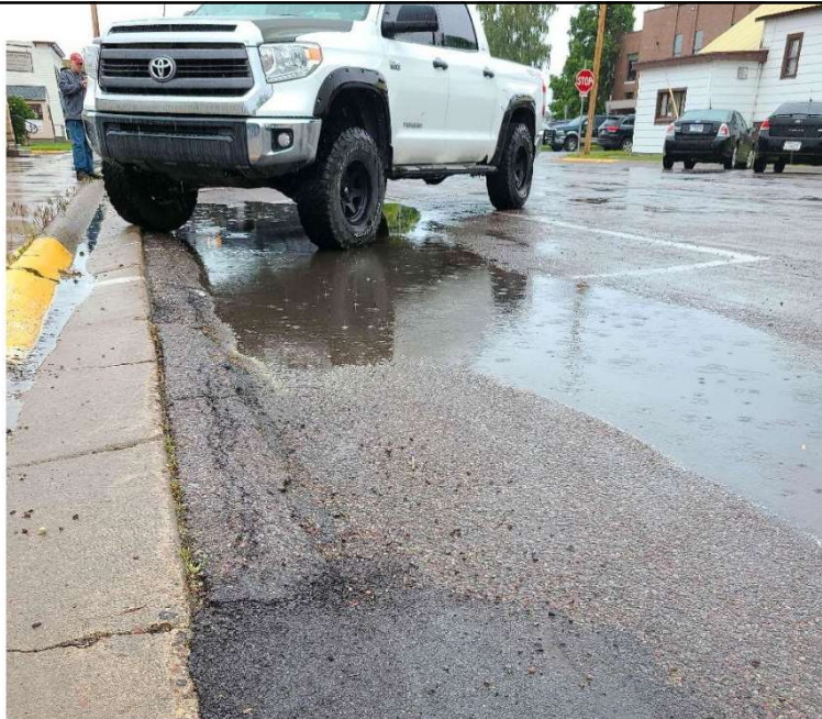
1 st Street E. – Curb and Subgrade Failure
