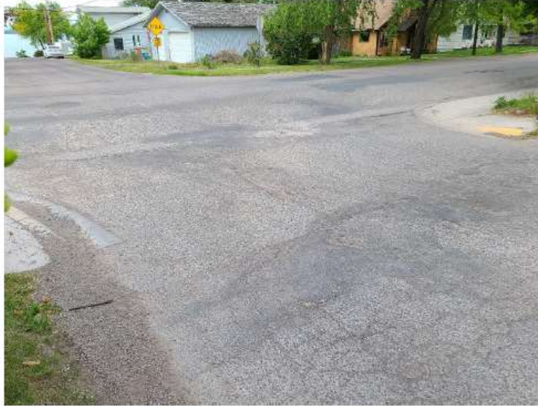
4 th Ave. and 7 th Street Intersection – Severe Subgrade Failure
