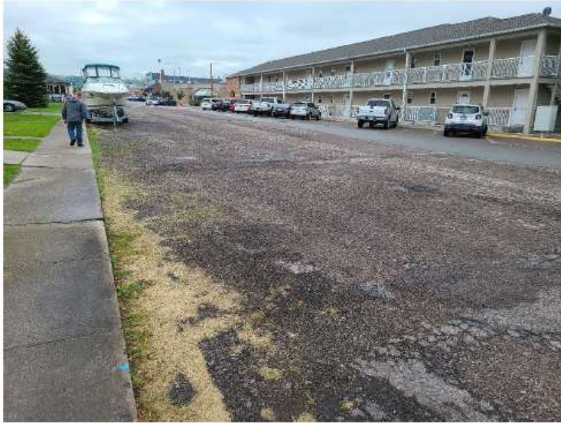
1 st Street E. – Pavement Deterioration
